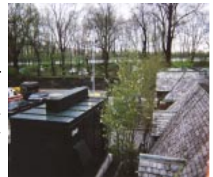
UTC Fuel Cells installed this 200-kW fuel cell power plant at the Central Park Police Precinct in New York City.
