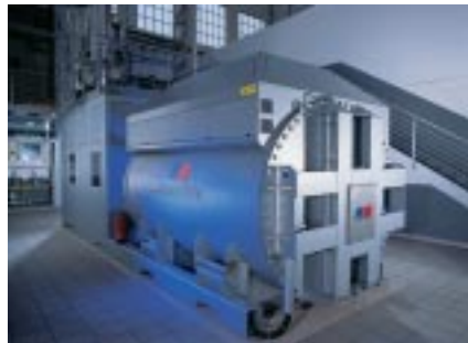
In 2004, FuelCell Energy's European partner, MTU CFC Solutions GmbH, plans to begin commercial sales of MCFC power plants, such as this one installed at the
